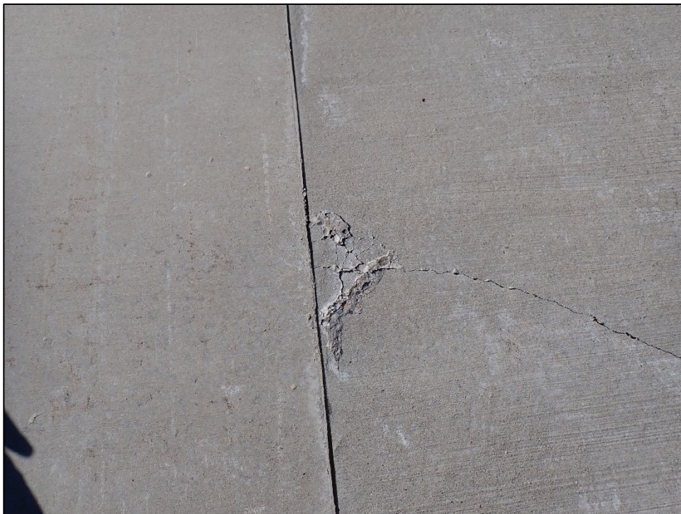
AP-22-02: Joint Spalling
