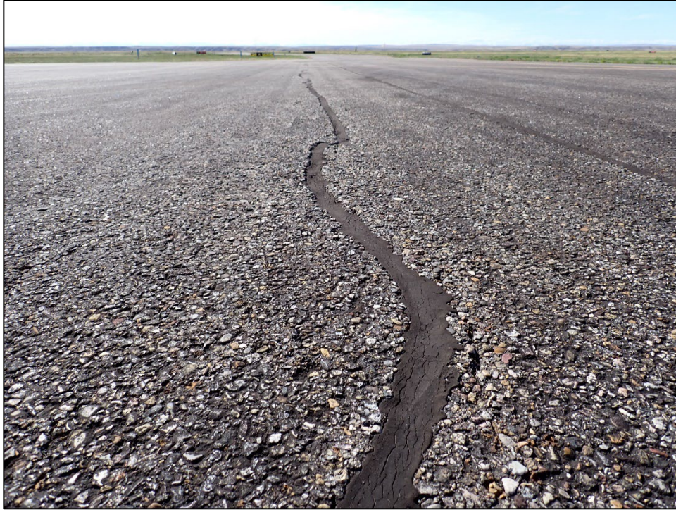
AP-21-20: L&T Cracking
