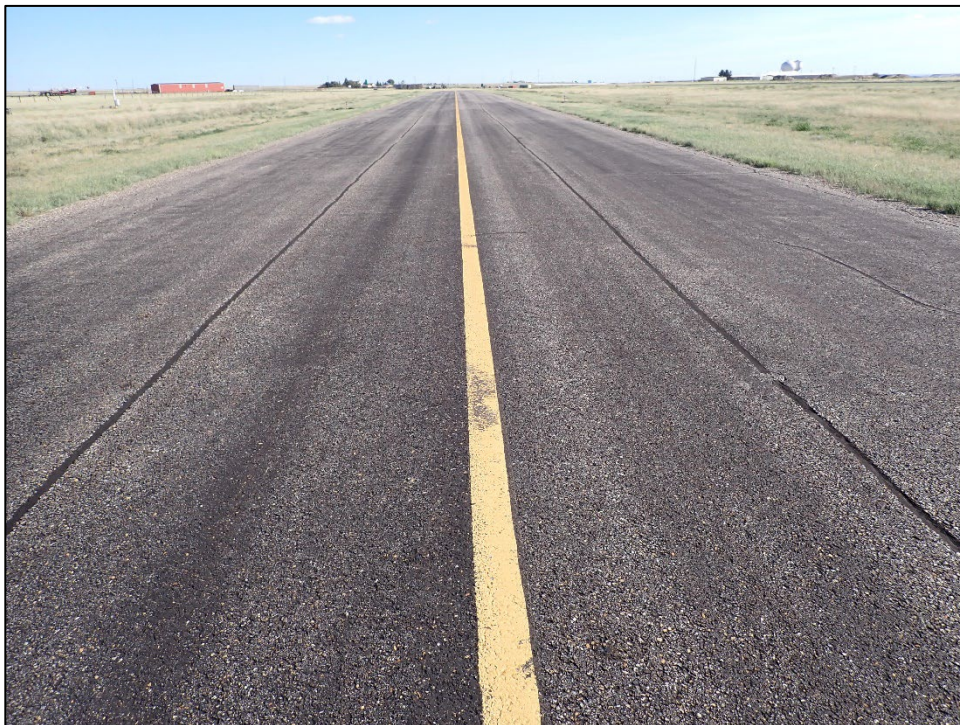
TW-21-11: L&T Cracking
