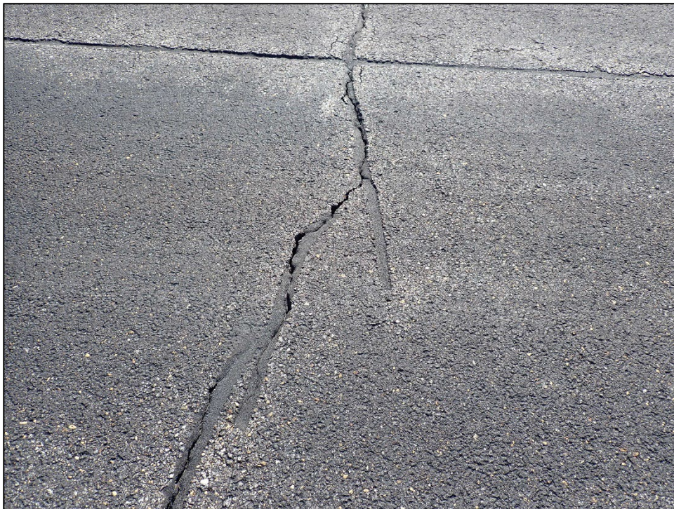
RW11-22-14: L&T Cracking
