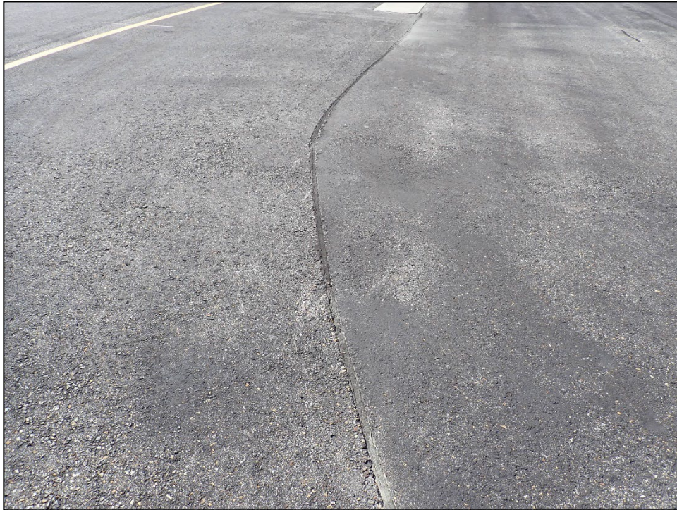
TW-17-06: L&T Cracking
